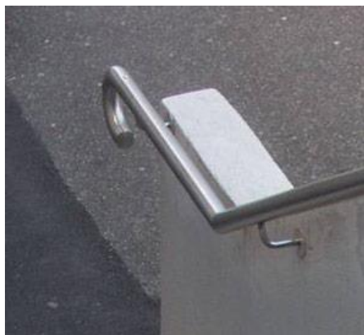
Figure 6.6: Rail extends beyond the stair.
