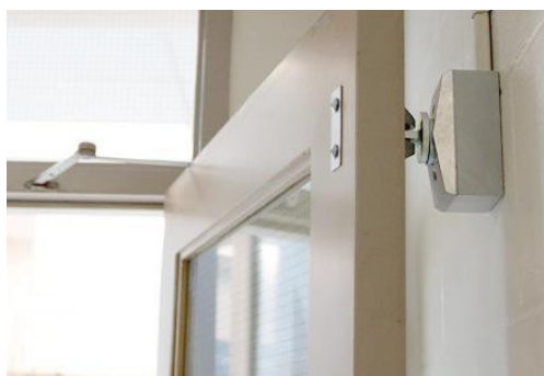
Figure 5.7: Electronic operated door hold open device
