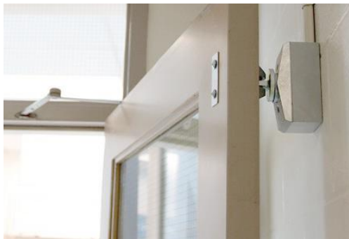
Figure 5.7: Electronic operated door hold open device
