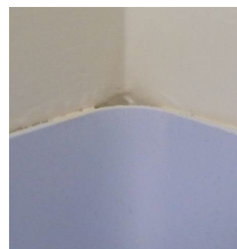
Gap between skirting and walls
