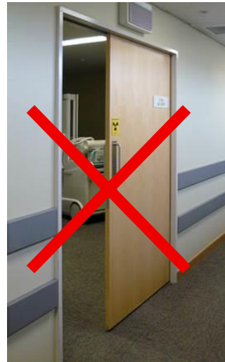
Figure 26: Cavity sliding doors not suitable for clinical areas
