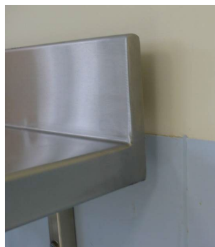
Gap between bench fitting and wall
