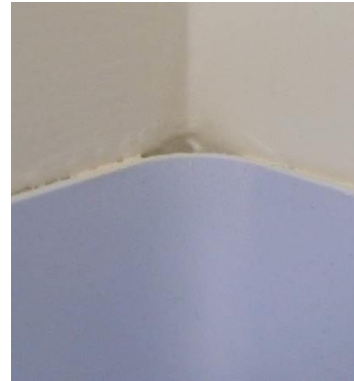
Gap between skirting and walls
