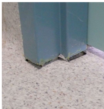
Figure 28: Gaps between door frame and floor
