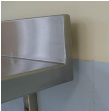
Gap between bench fitting and wall
