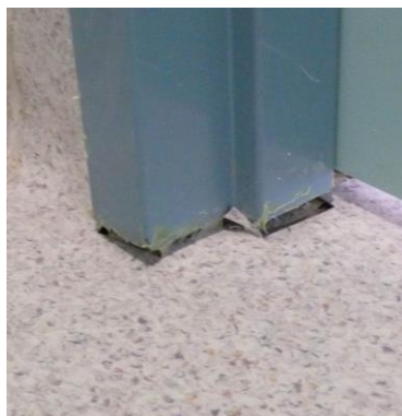
Figure 28: Gaps between door frame and floor
